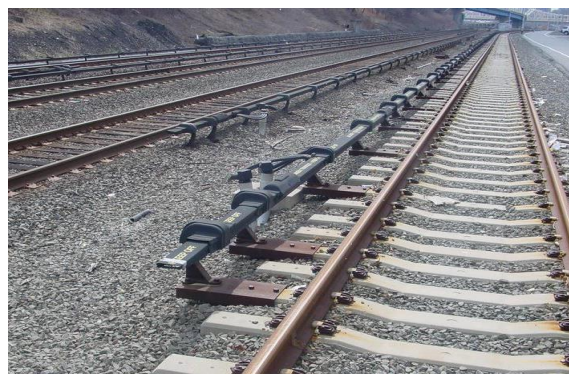
Fig. 2. A third rail system
